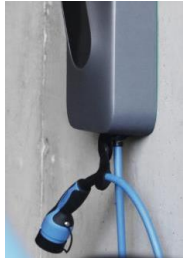
Figure 2: Private charging point with wall-box Source: ETREL
