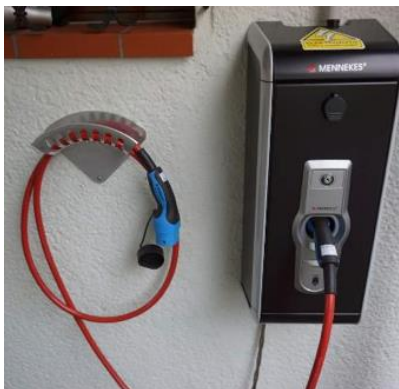
Figure 6: Private charging station - always available and using ones own power Source B.A.U.M. Consult
