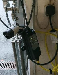
Figure 1: Home charging with cable control box (ICCB) Source: B.A.U.M. Consult
